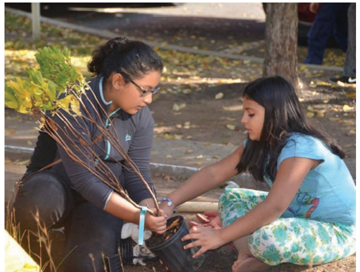
Community members and elected officials plant a rain garden in the Town of Harrison, as part of the Passaic Valley Sewerage Commission’s green infrastructure program.
