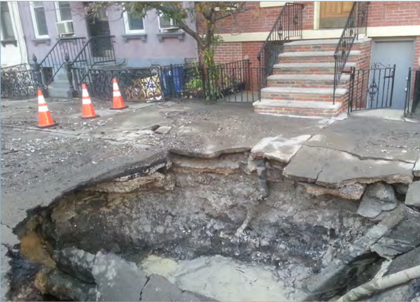
Water main breaks force the closure of roads both during (top) and after (left) the event. The stresses on a water main from a service interruption and restoration are enough to trigger additional breaks along the line.
