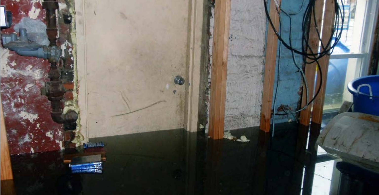
Like those of many of his neighbors, Tom Chartier’s basement was hit hard by Hurricane Irene and Superstorm Sandy. While in Tom’s case Hurricane Irene flooded an unfinished basement in the process of renovation (as seen in the picture), the subsequent repairs and renovations were almost completely washed away by Sandy. Photo credit: Tom Chartier.
